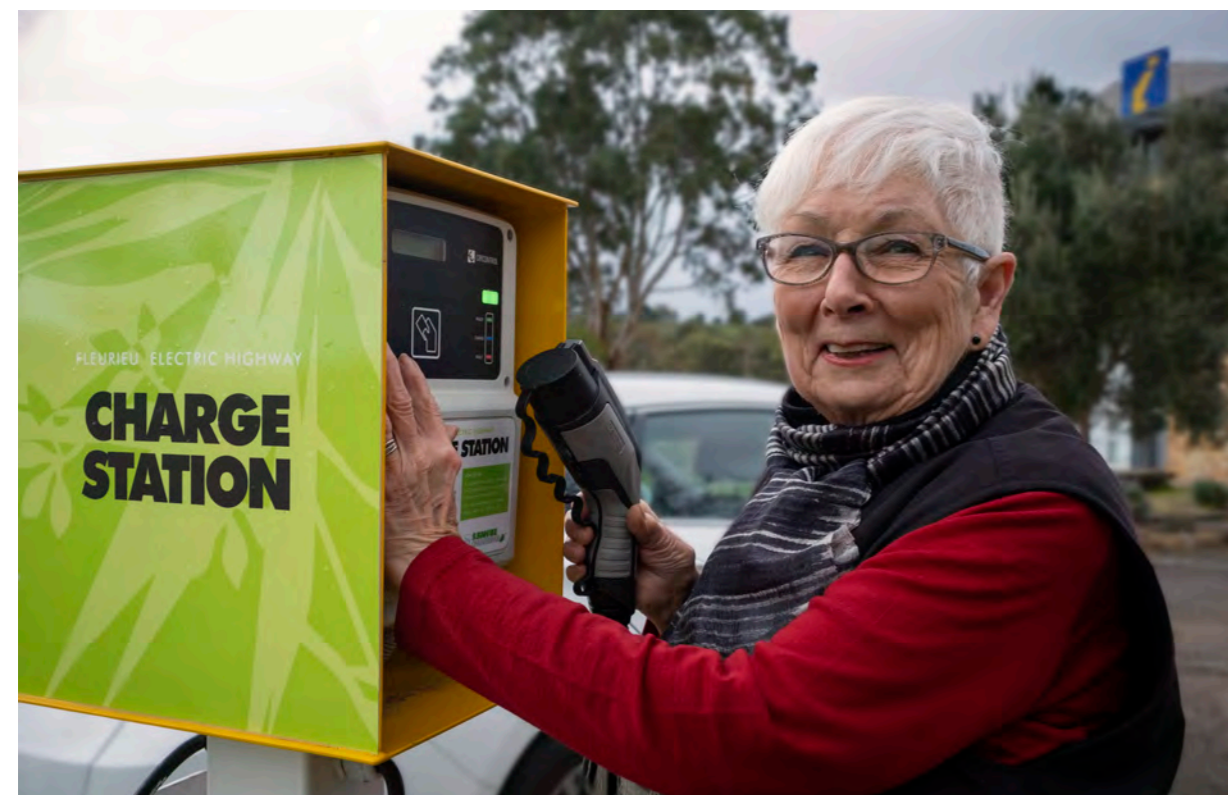
Electric vehicle charging infrastructure at the McLaren Vale Visitor Centre
